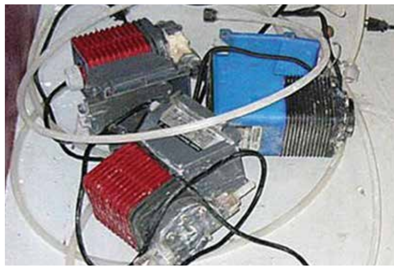
Solenoid-driven diaphragm metering pumps often become vapor-locked from NaOCl outgassing and jammed due to crystallization.
